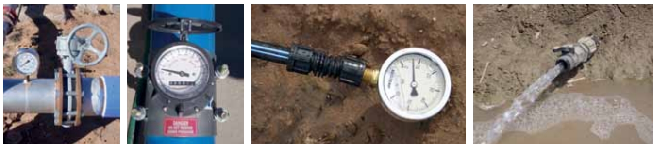
From left to right: Pressure gauge on mainline; flow meter; pressure gauge on tape; monitoring tape flush water.
